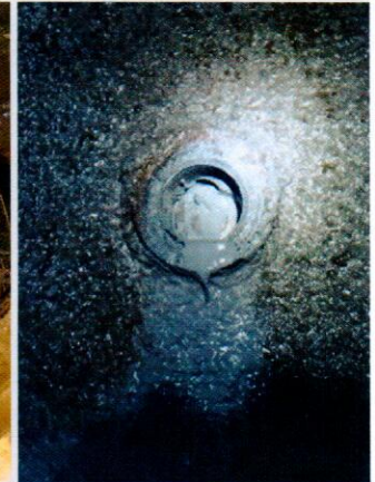
The grouting material is leaking out from an expansion hole
