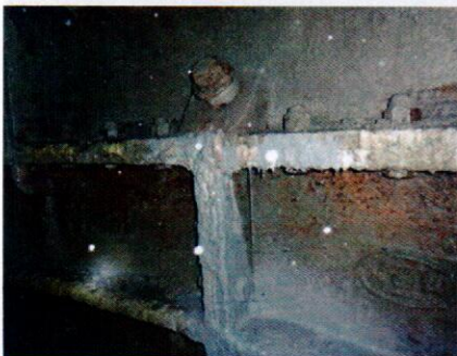
Grouting material is leaking out of the tubing joints- a sign of effective grouting
